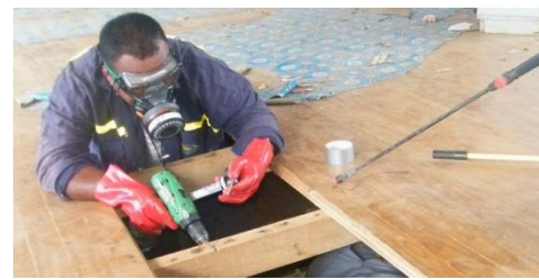
Termite officers remove damaged flooring to treat for AST infestation
