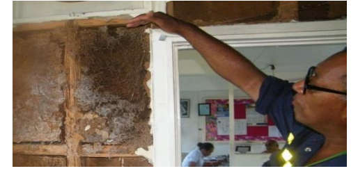
AST damage on the inside of walls at an office building in Lautoka
